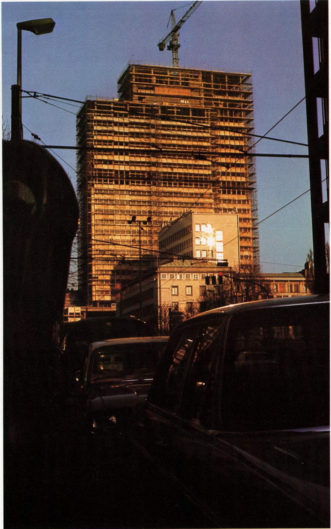
The shell of our new high rise Frankfurt headquarters was completed at the end of 1972.
