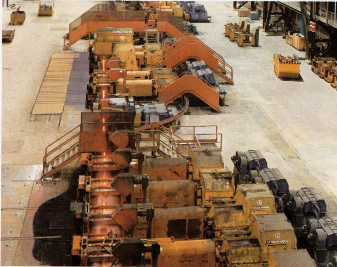
Schloemann AG is erecting a fully automatic light-section rolling mill for the ISCOR steel concern in South Africa. Commerzbank has a part in the financing of the project.
